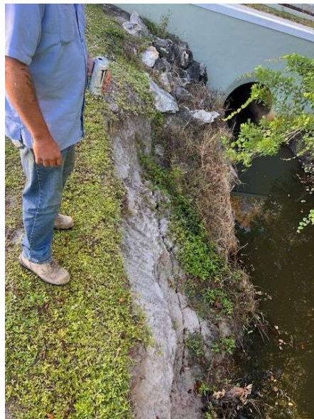
Before Caving Into the ditch
