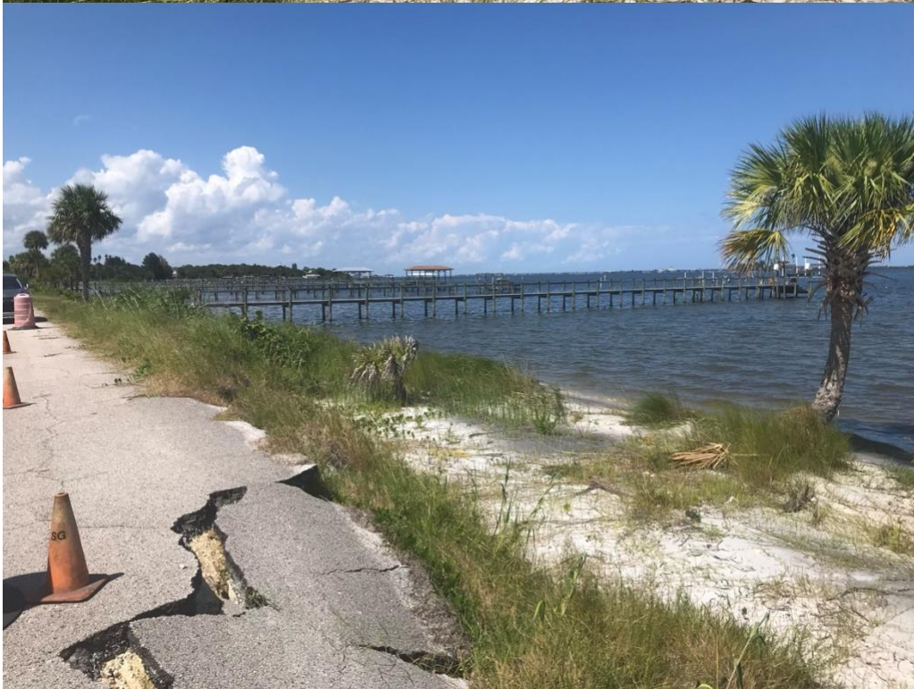
Figure 2. Recent damage to the road and shoreline on Rocky Point Road.
