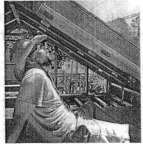
SENIOR LIFE Photo Rob Hayward enjoys the fruits of his labor after installing a roof window in the loft of his tiny home.
