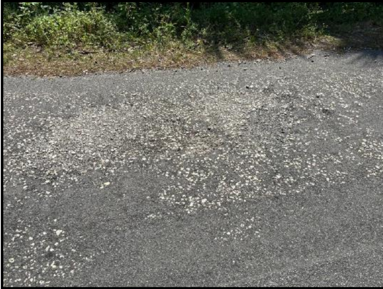
WEATHERING AND RAVELING OLD MISSION ROAD
