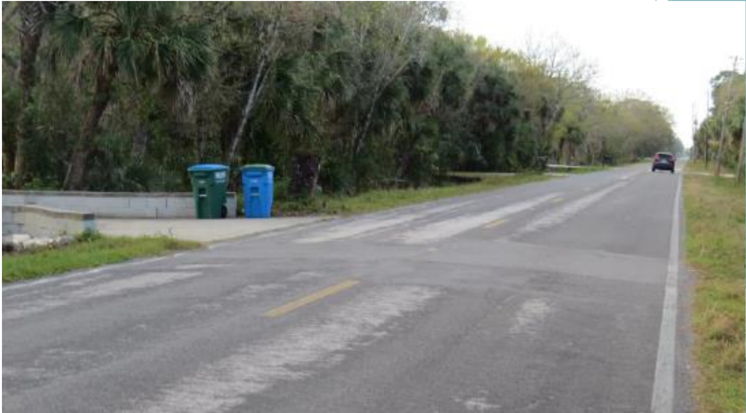
RUTTING AND DEPRESSIONS WEBER ROAD
