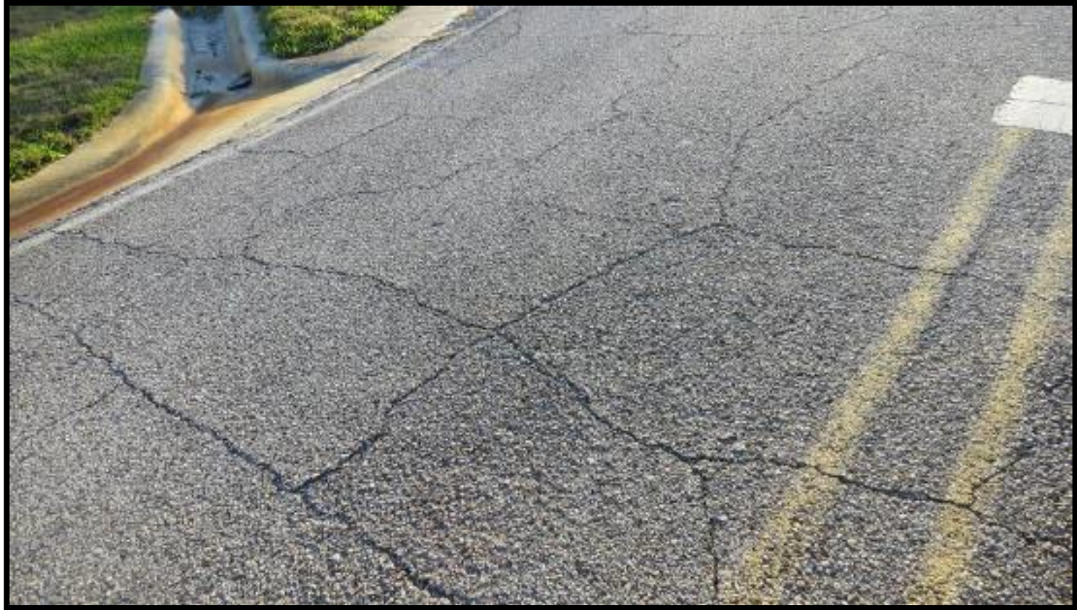
BLOCK CRACKING FALLS TRAIL
