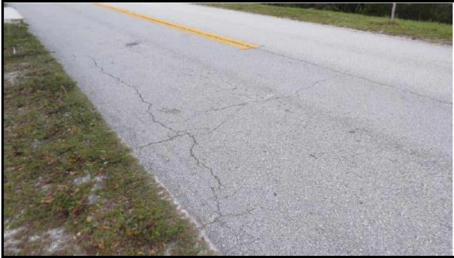
LONGITUNDINAL AND TRANSVERSE CRACKS COREY ROAD
