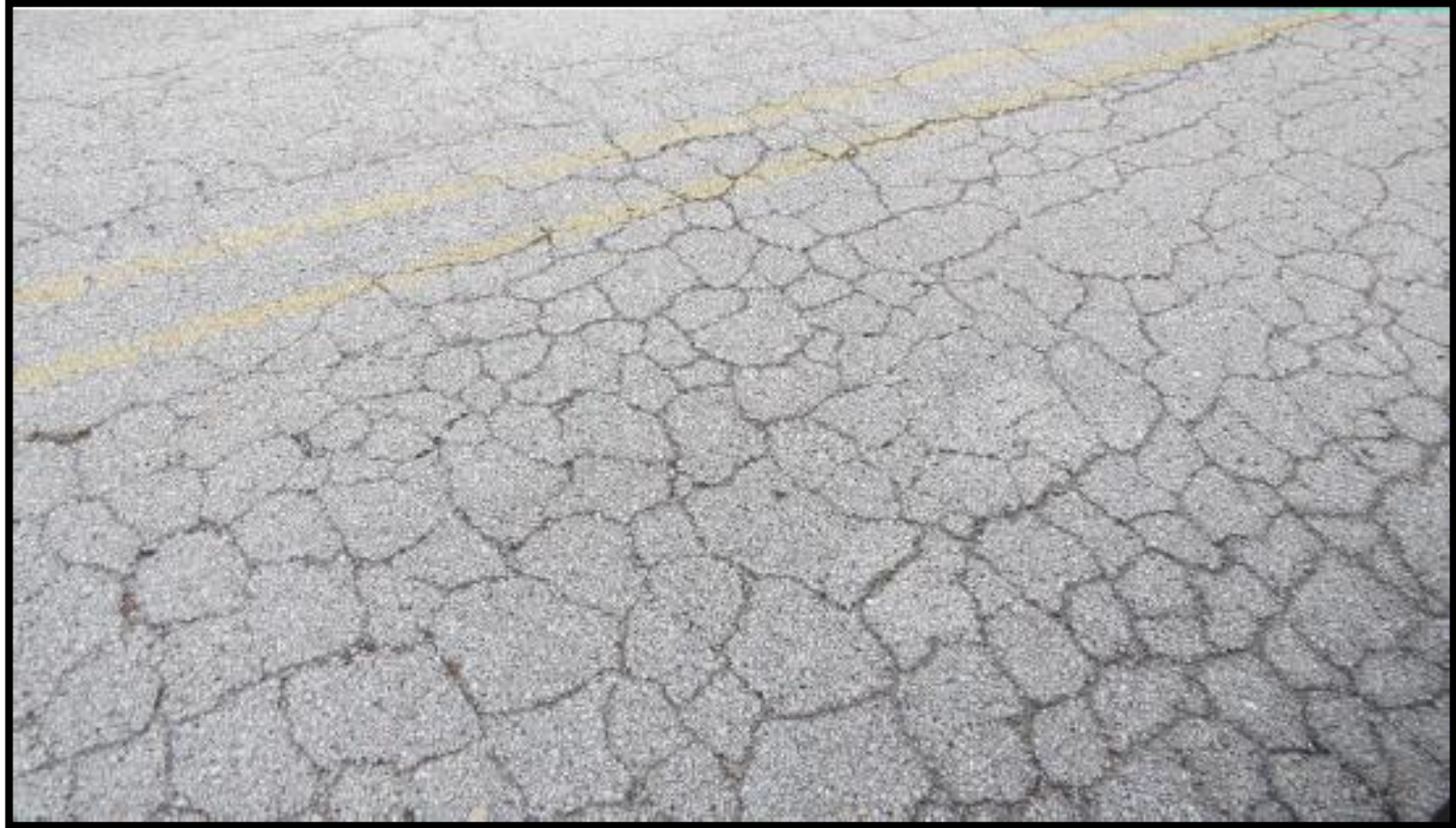
ALLIGATOR CRACKING CORAL WAY
